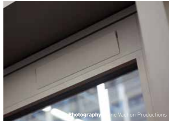
Access hatch for maintenance.
