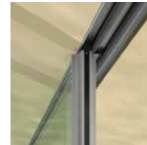
View of the open pane, showing upper frame built into the false ceiling.
